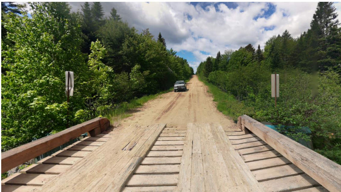
Figure 4-4 Wooden Bridge above a creek noted along Bronson Settlement Road (Google Maps, 2024)
